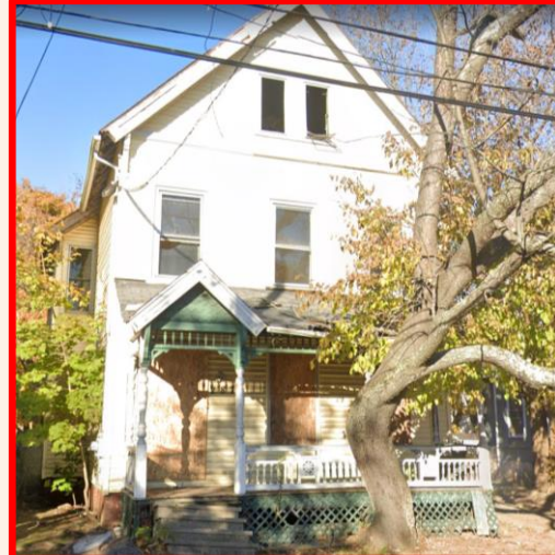
287 Division St Vacant home
